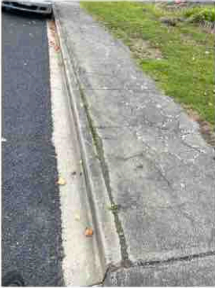
71. Contractor damage outside 17 Pounamu Rd
